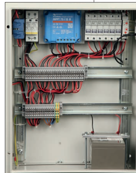
Battery box + charge regulator.
