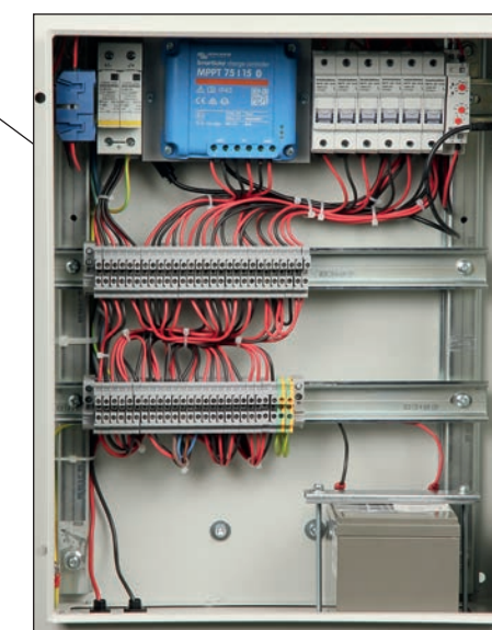
Battery box + charge regulator.
